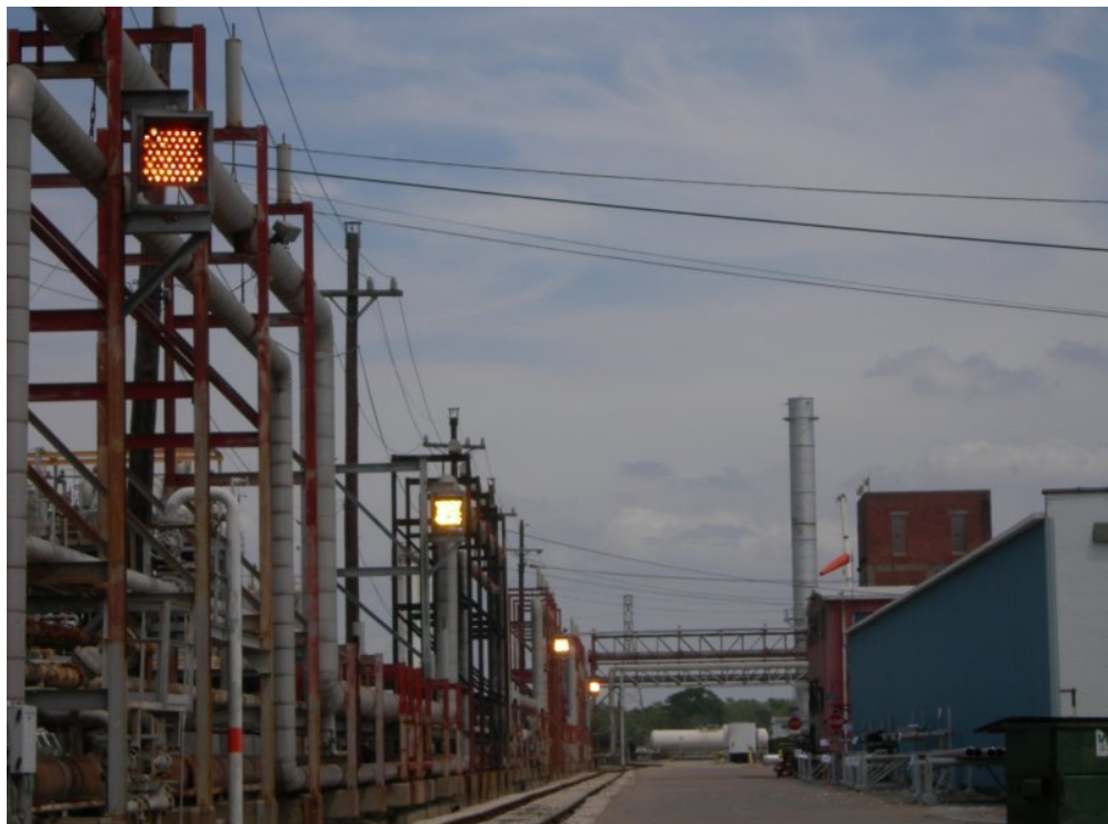
Retro arrays on the North boundary of Texas Petrochemicals. Retros are mounted on the pipe chase and appear illuminated because of the flash of the camera.
